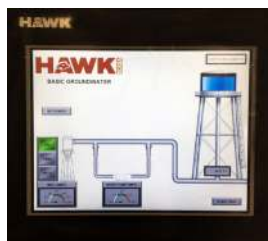
HMI touchscreen panel for onsite monitoring & controlling
